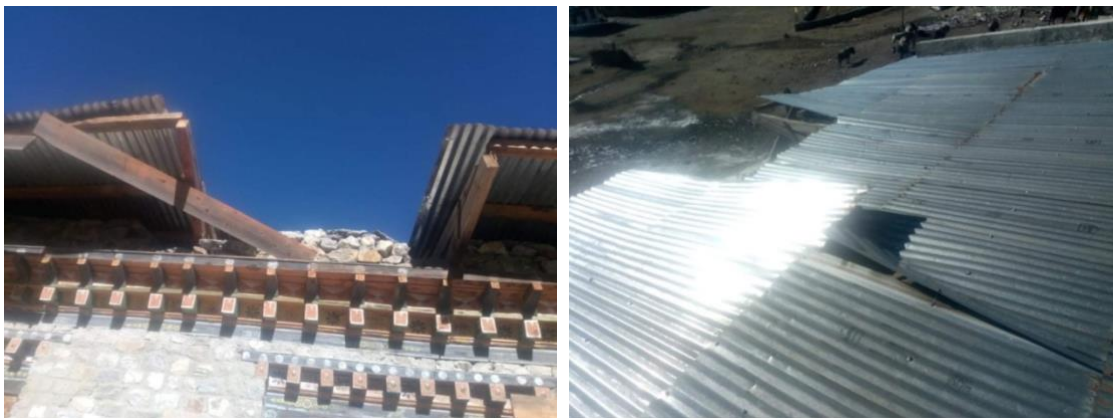
Fig 12: Room of Soe Park Range damaged by windstorm
