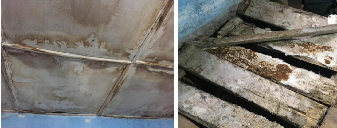
Fig 13. Ceiling and floor damaged by down pour penetrated through damaged roof
