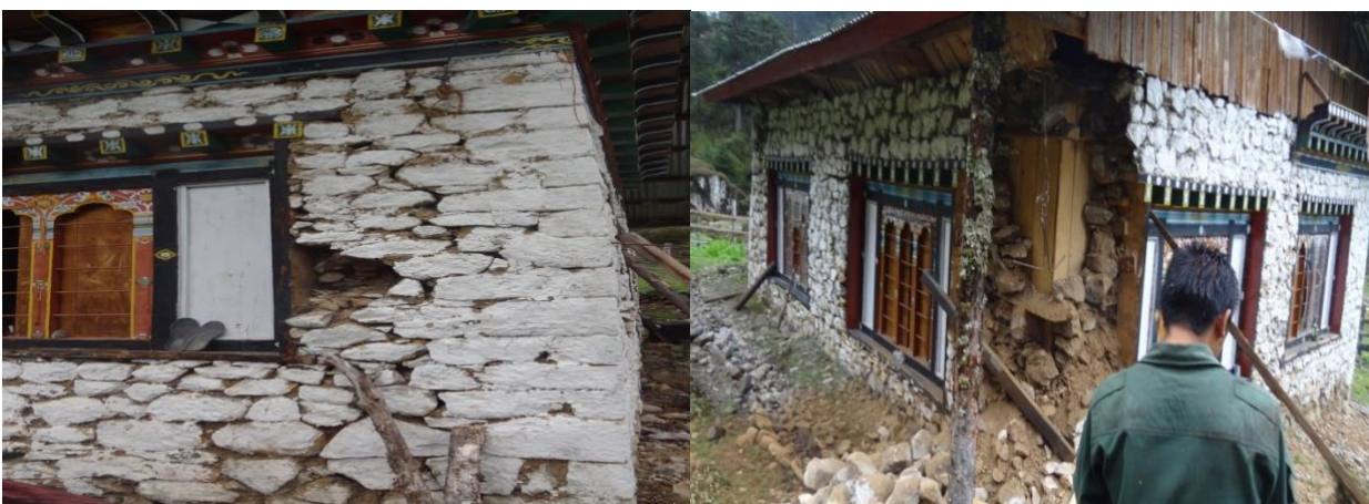
Figure 5: Condition of BWS office structures
