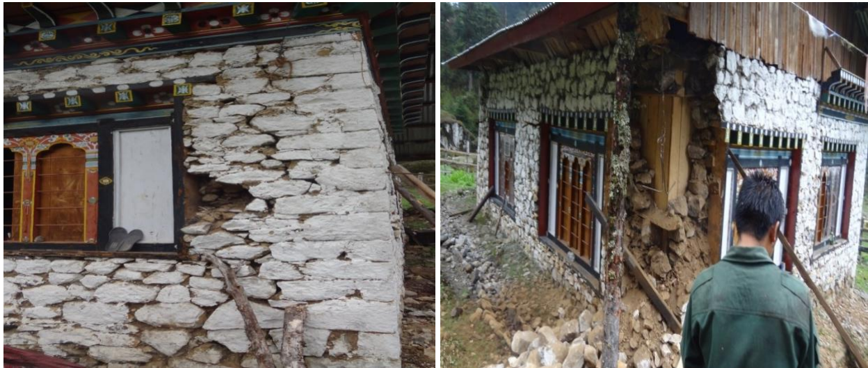
Figure 6: Condition of BWS office structures
