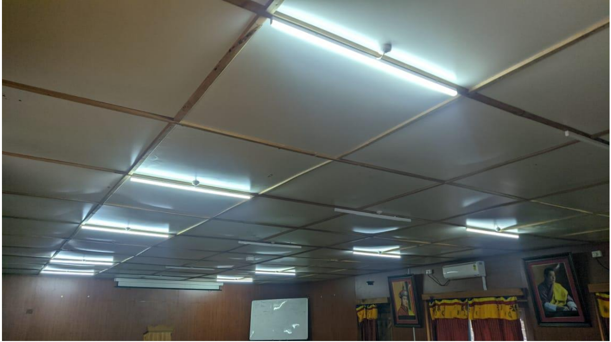
Good quality of ceiling and lighting work at Royal Botanical Park, Lampelri
