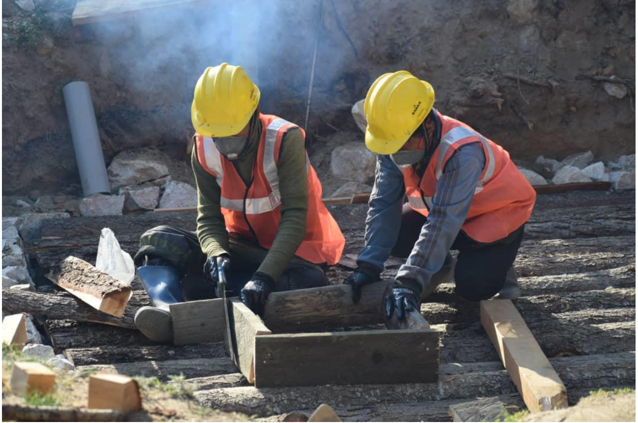
Use of safety gears by workers during the construction of toilet in BC2 under Khotokha Range Office
