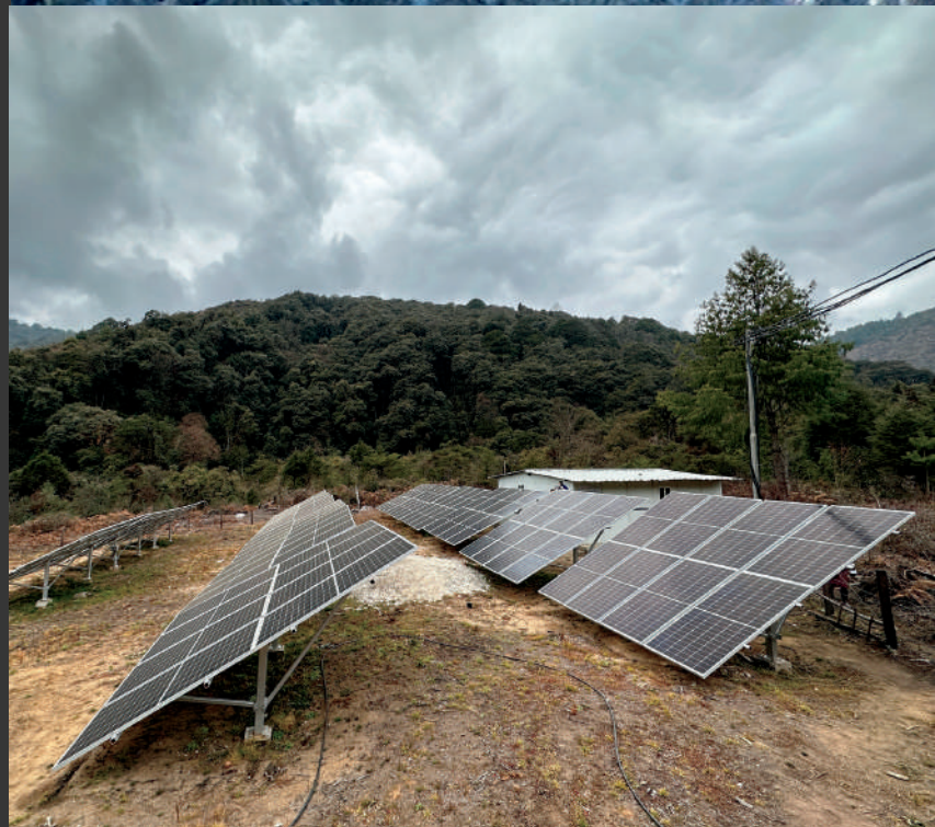
Photo 38: Solar Panel at Aja Nye (Dawathang)
